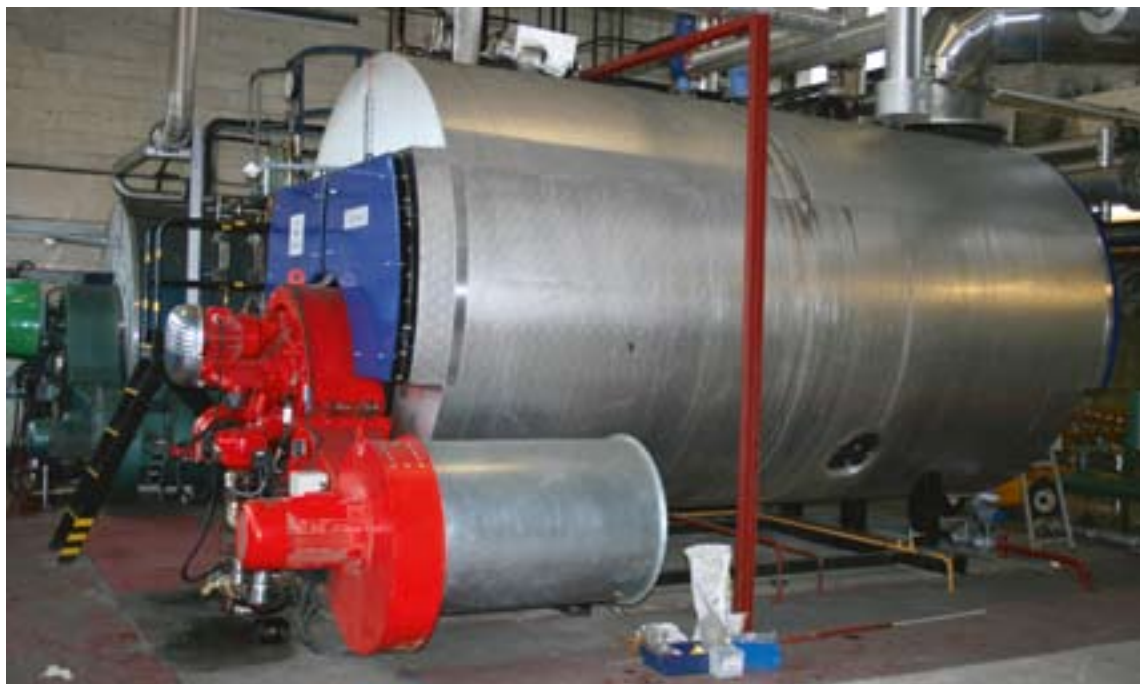
■ An oil fired boiler in the new energy centre
