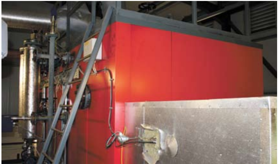
■ The new biomass boiler within the energy centre at Pilgrim Hospital, Boston
